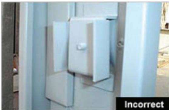
The pressure anchor that has not been properly adjusted. The adjusting screw has not been loosened in order to move the pressure anchor back against the frame.
